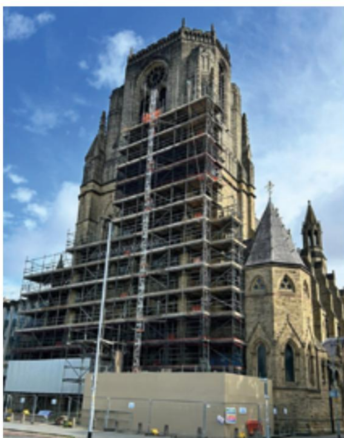
Scaffolding for the tower work in front of Holy Name church, August 2024
