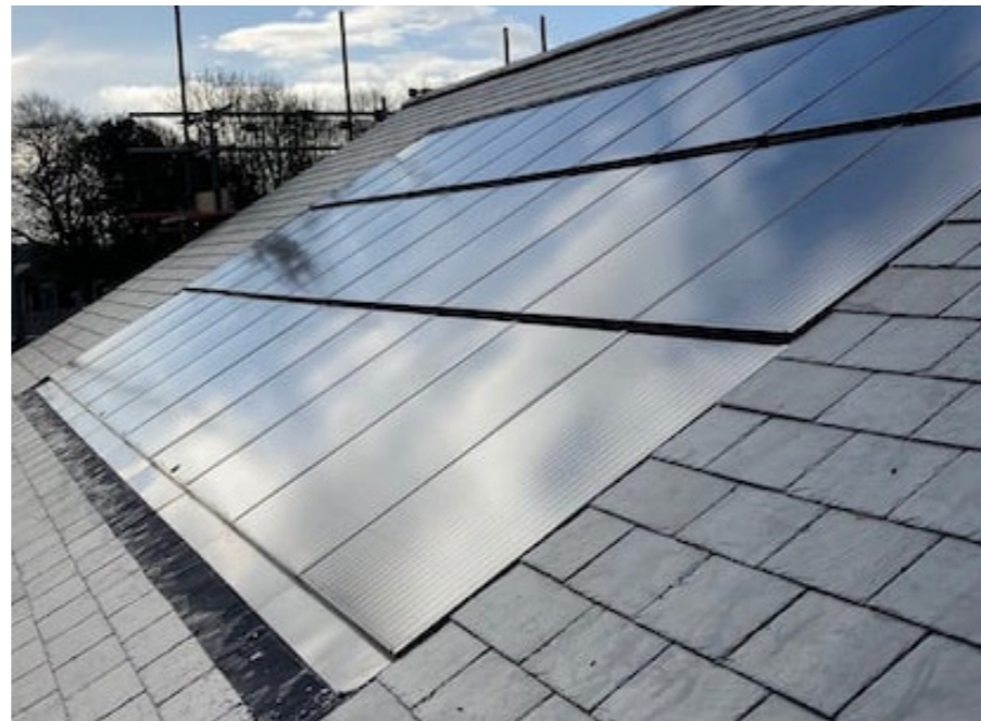
SOLAR PANELS Integrated into the design of the new slate roof.
