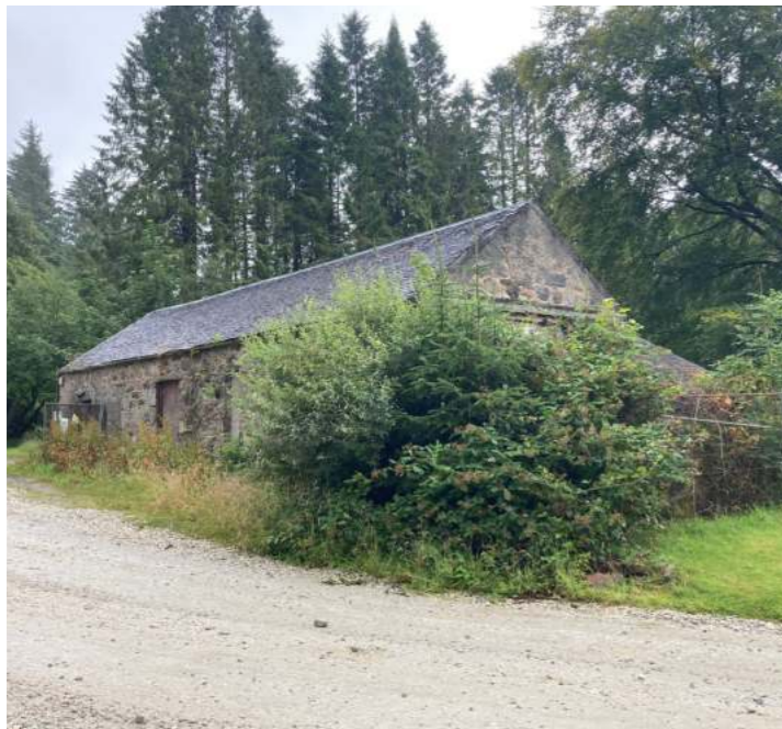
SHRUBS TAKING OVER THE BUILDING
