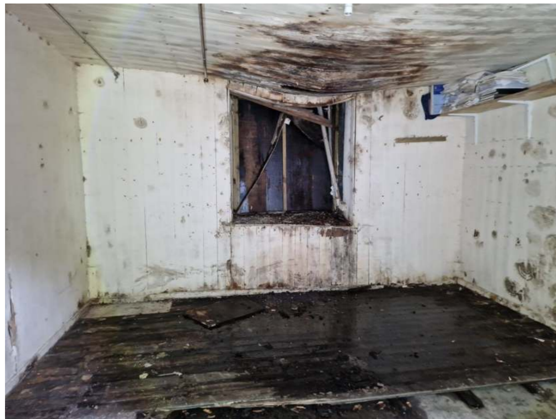
Fig. 18 – An example of the interior water damage.
