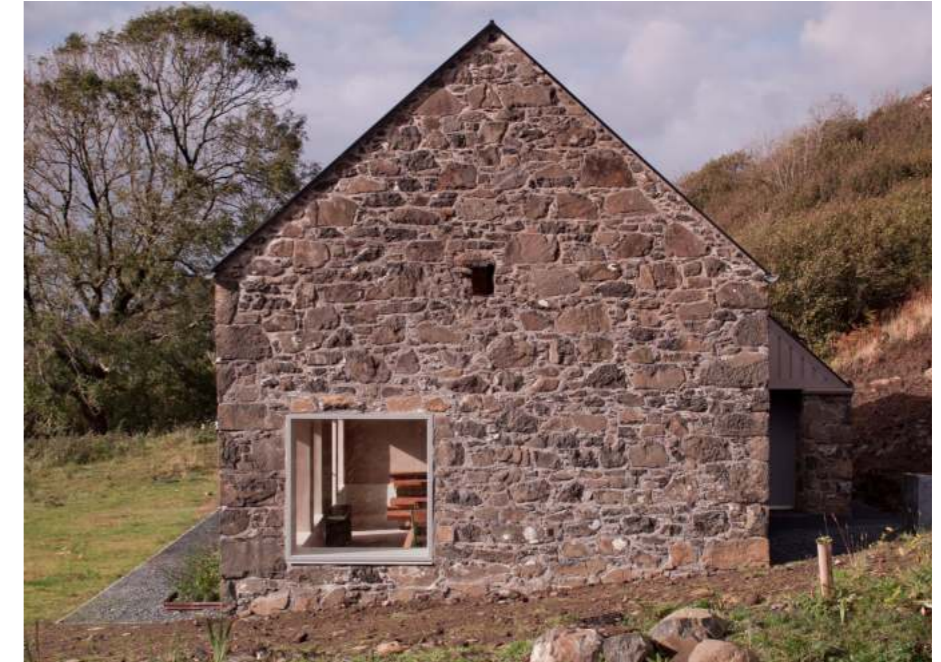
RETAINING EXISTING STONE Used to create texture and reflect traditional techniques. (Croft 3, Fardaa)
