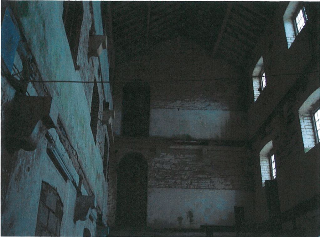
Internal view of male dormitory. The mullions are clearly visible on the left hand side which held up supports for the floors.
