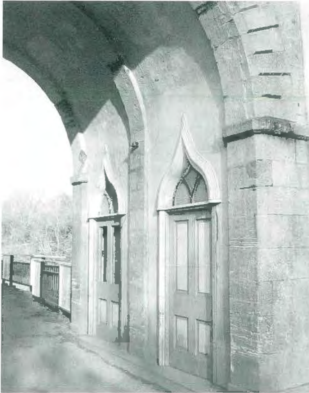
Figure 4: Interior of archway, demonstrating vaulted ceiling through the archway and symmetrical ogee headed doorways.
