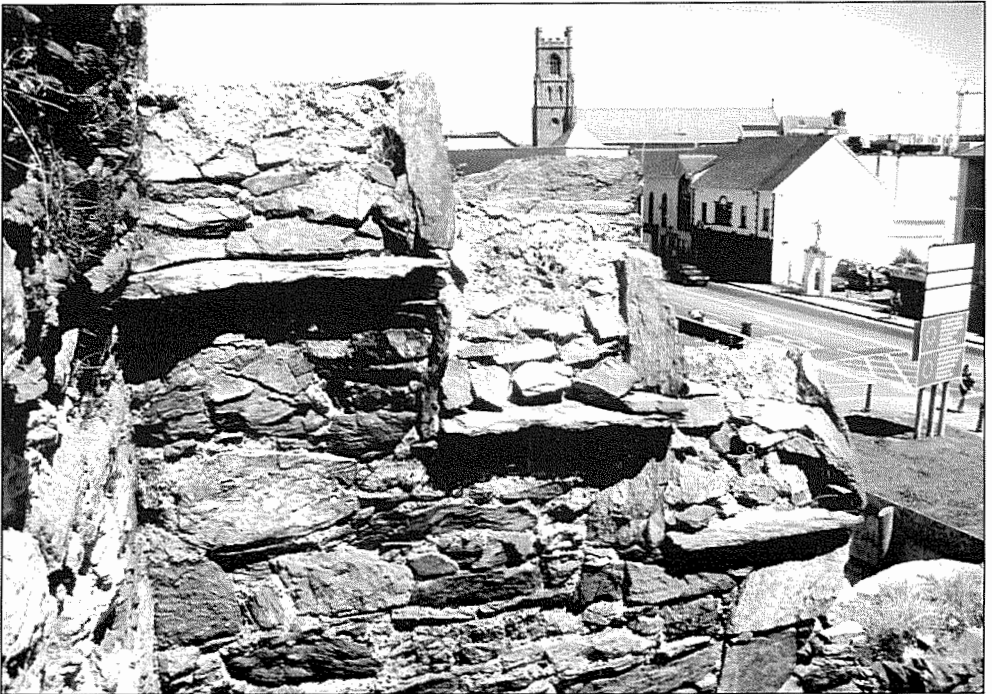
Plate 10 - Rare example of original stepped crenellations on top of city wall at southeast end of Double Tower. BM July '04.
