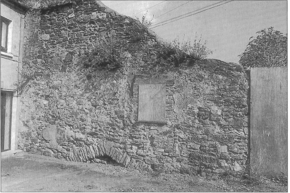
Plate 3 – Top of the main archway (Arch A) into the Watergate as viewed from Mendicity Lane.
